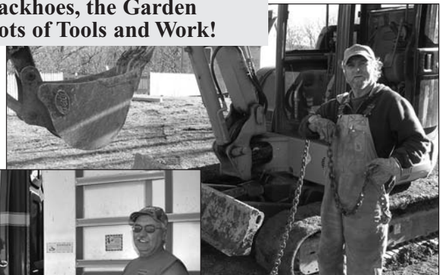
Above Right: Roy "Butch" Green from GRC helped excavate and level the new garden site.
